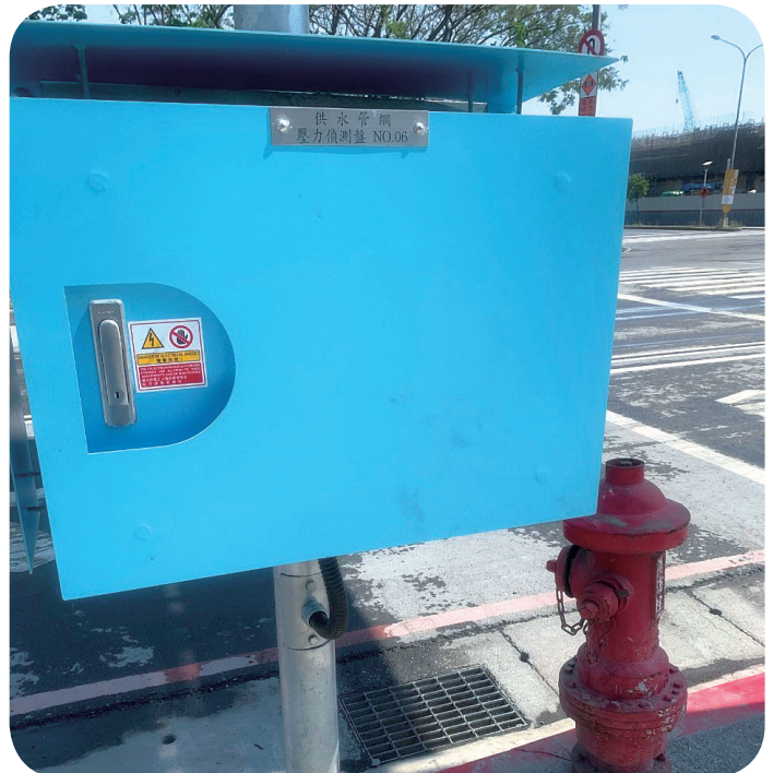
Monitoring Equipment for Pressure on Water Pipeline Network
