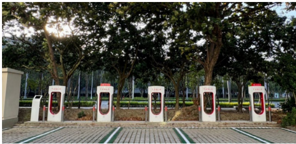
(Left) Park17 electric vehicle charging station
