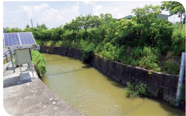
Water level monitoring installation
