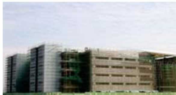
Figure 5-6-13 Lujhu Science Park's Phase 1 Standard Factory ( to be completed in June 2004 )
